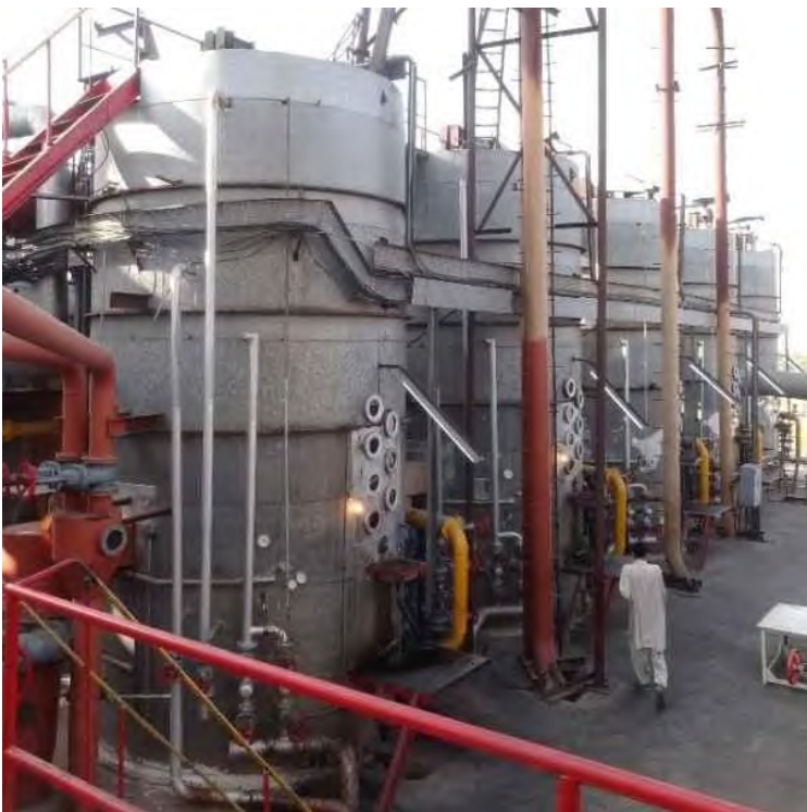
Cascade plus in operation at Almoiz Industries Ltd., Pakistan
